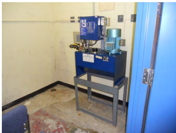
Photo #27: Elevator equipment
