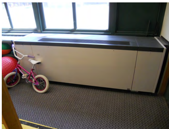
Photo #30: New univentilator
