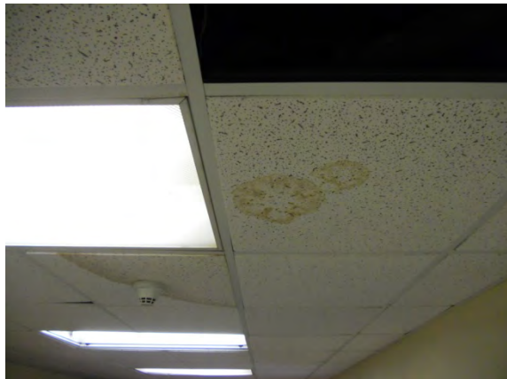
Photo #25: Water staining
