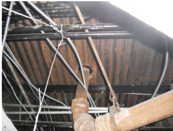
Photo #26: Drain line above stained ceiling tiles
