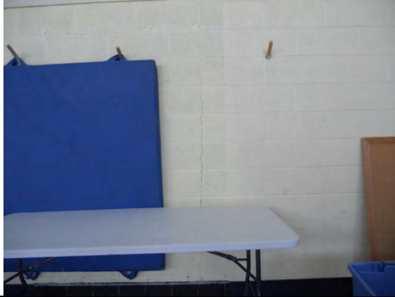
Photo #43: Cracking in gymnasium
